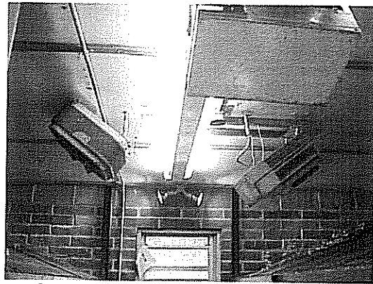
Same barn with 8' fixture and 2 pairs of flood lights
